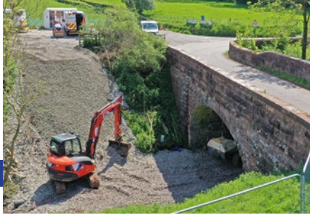
A photo capturing the extent of progress with the infill works on 1 June 2021.
