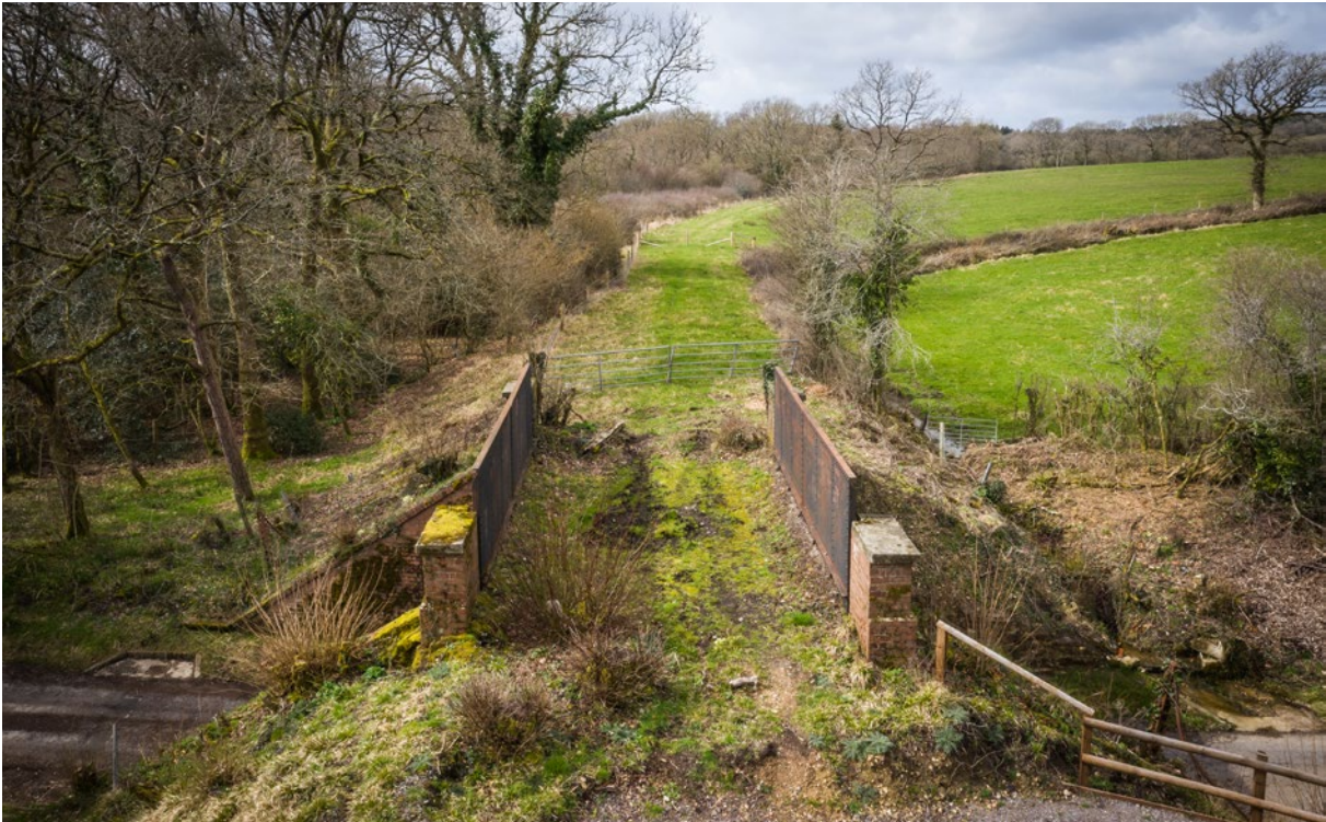
Demolition of the bridge would impose significant additional costs on any future active travel or rail scheme involving the former Bridport Railway.
