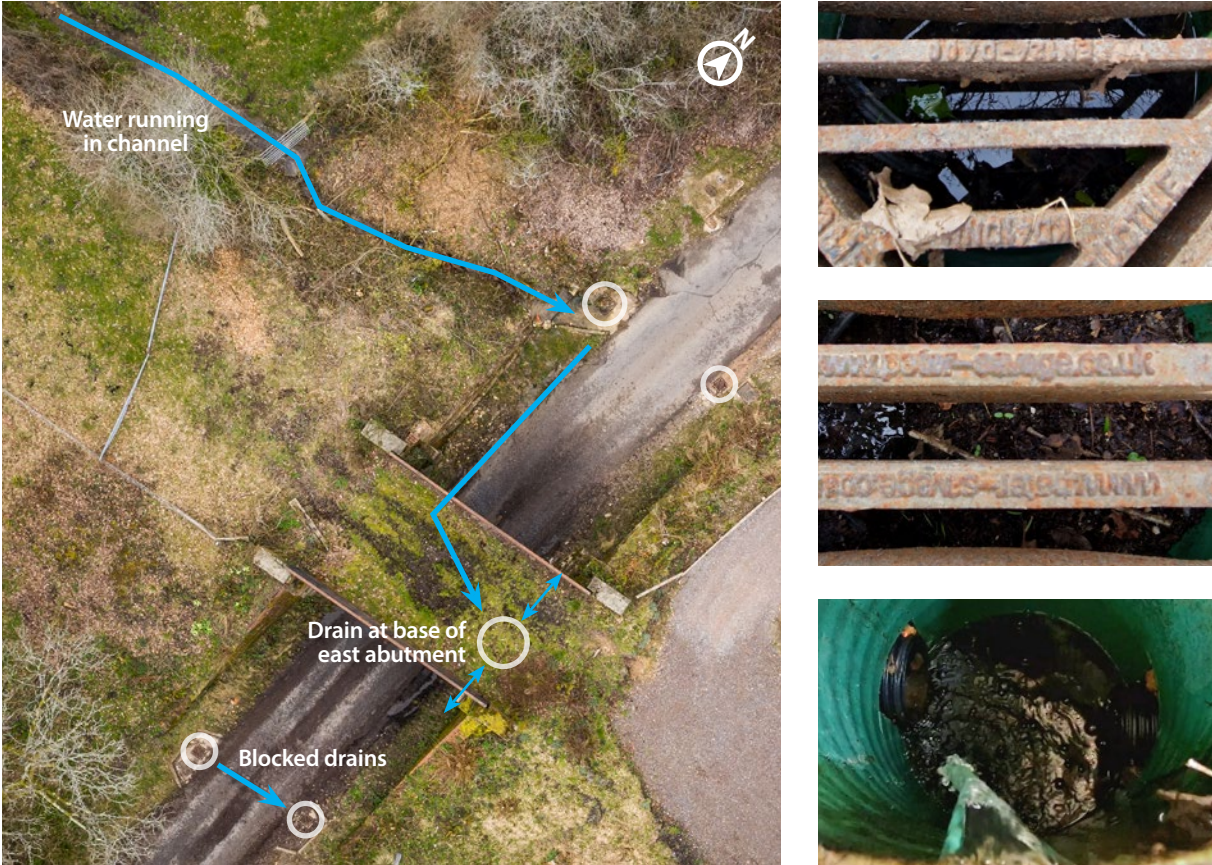
An overview of the bridge drainage system, with additional views into the south-west drain (right upper), south-east drain (right middle) and abutment drain (right lower).
