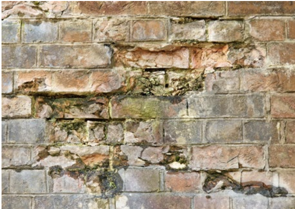
Figure 5: Degradation of the east abutment.
