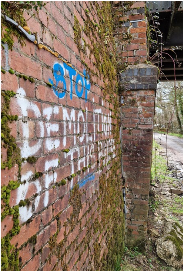
Figure 4: Rotation of the east abutment.
