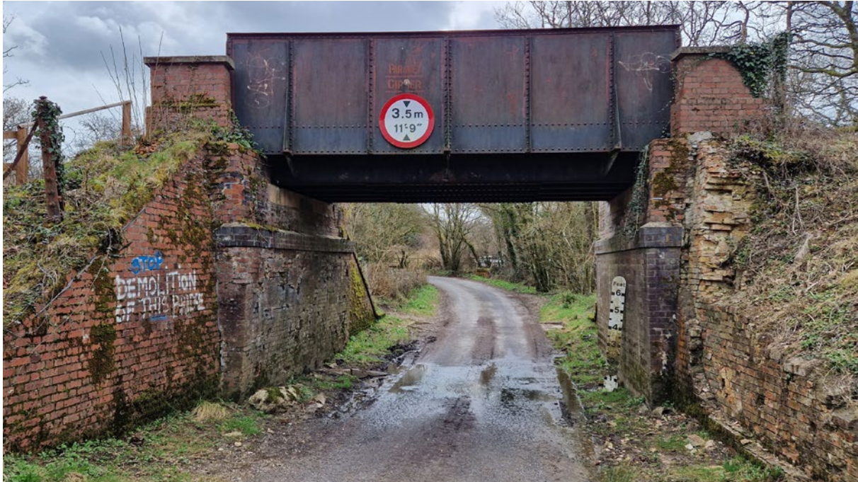
Figure 1: The bridge's north elevation with sign indicating the height restriction.
