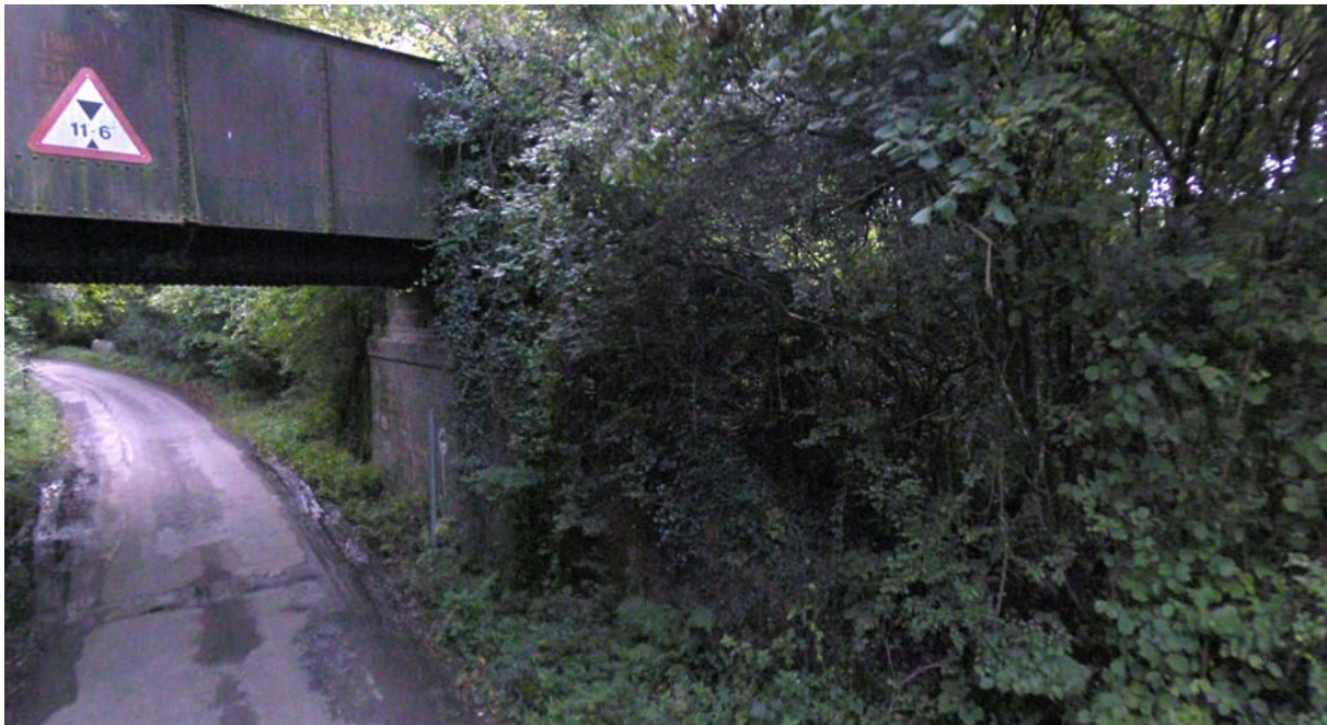
Figure 6: 2011 photograph showing extensive tree growth around the north-west wingwall. (Google Streetview)
