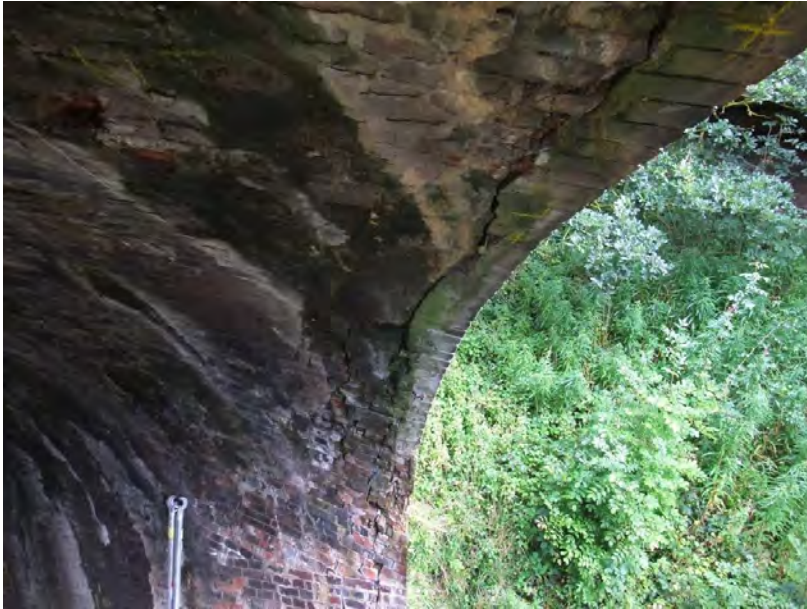
Figure 6.4: Damage to brick bridge at Great Dunchurch. Cyclic live loads have caused a crack to develop through the ring where the spandrel wall stiffens the edges.
