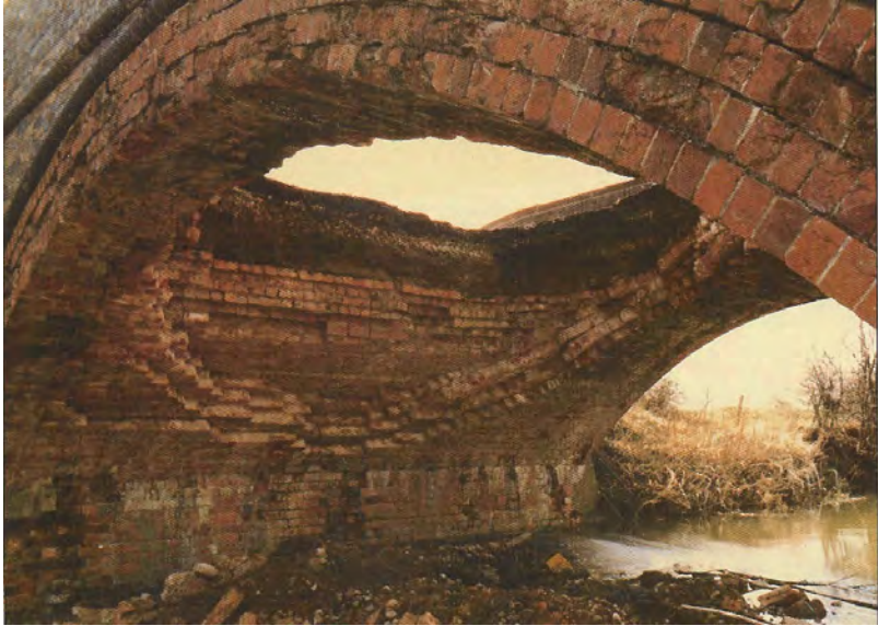
Figure 6.1: A masonry bridge in which the arch ring dropped out.
