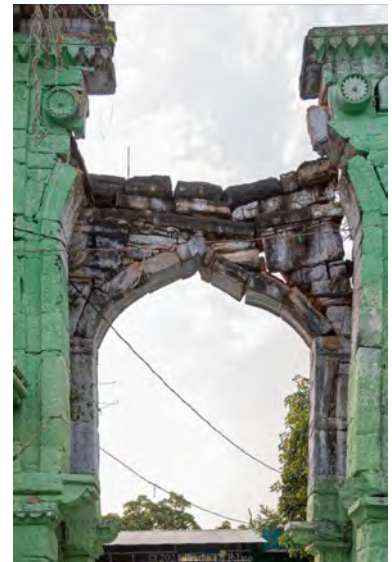
Figure 6.2: Impending collapse of a decorative stone arch, showing the degree of abutment movement required to allow this.
