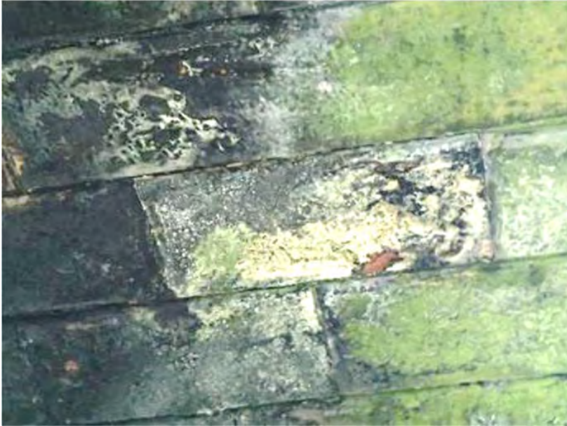
Figure 2.2: Photo 12 from 2020 visual, showing dropped stone. Quality is limited but exposed edge does not look at all different. We would expect a cleaner face in a recently dropped stone, and abrasion or damage in a stone dropping due to mechanical action.
