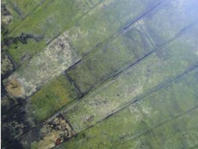
Figure 2.4: Example of open joints, presented as photo 14 in 2020 visual inspection report. The voids are over limited lengths of joint; there remains ample area to carry the thrust.
