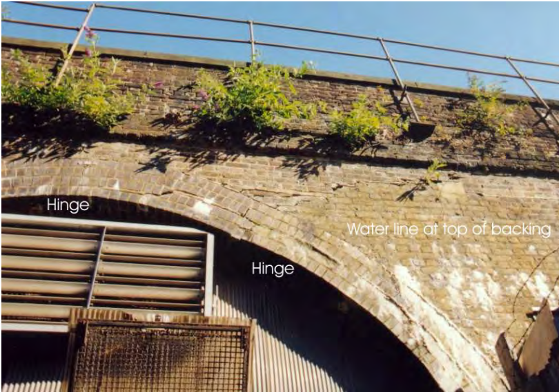
Figure 6.3: Damage resulting from a pier dropping around 100mm. The structure continued to carry rail traffic without risk of collapse.
