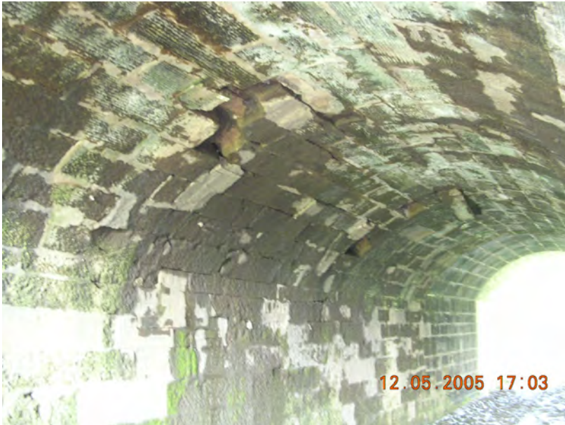
Figure 6.6: Severe damage to a bridge, with stones dropping due to mechanical action.
