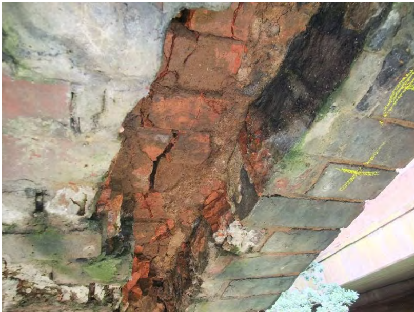
Figure 6.5: Here, the crack has bifurcated, creating an island patch which has then fallen out.
